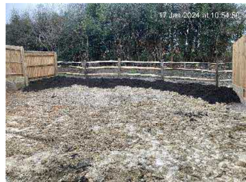
Plate 6 – Example of topsoil being placed in plot 174, marks on fence posts indicate 150mm topsoil has been placed, taken by the client 16/01/2024.
