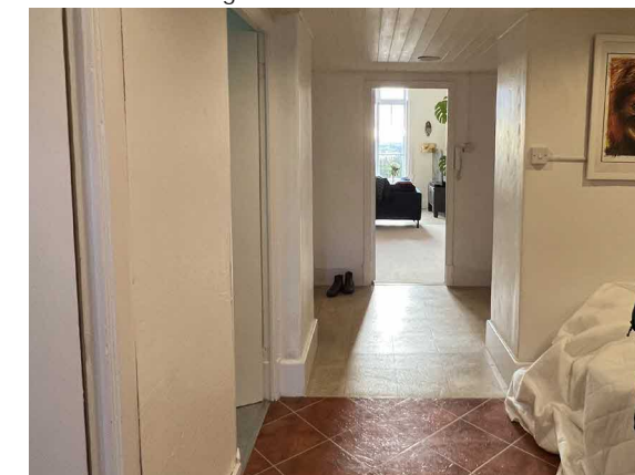
Entrance hall with false ceiling and modern partitions on right hand side.
