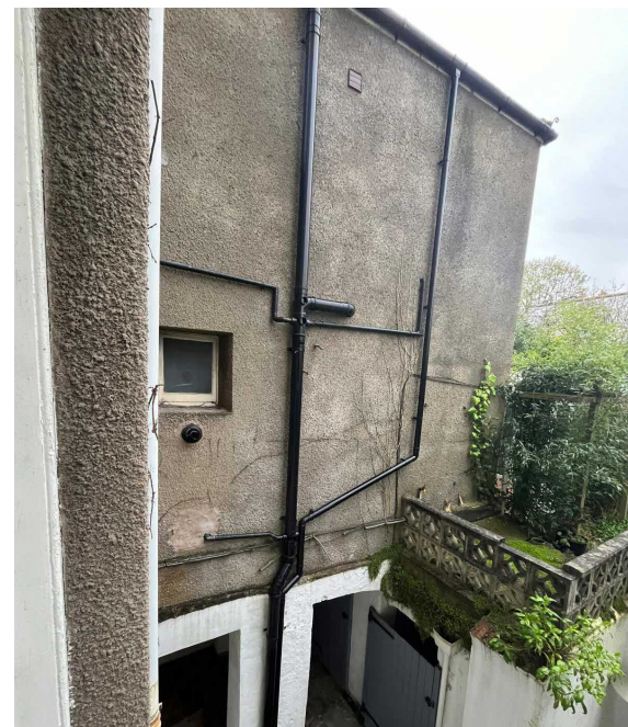
Existing side elevation to rear outrigger. Pipework to be rationalised.
