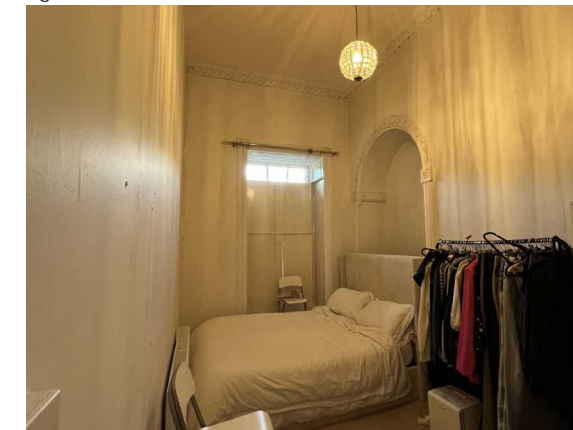
Existing bedroom with original floor-ceiling height and cornice. Modern partition on left hand side with no cornice. Original arched alcove with architrave detail.
