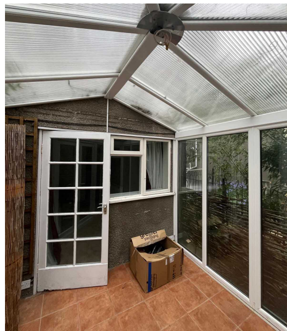
Existing white uPVC conservatory - opening resized to create new widened access through to new extension.
