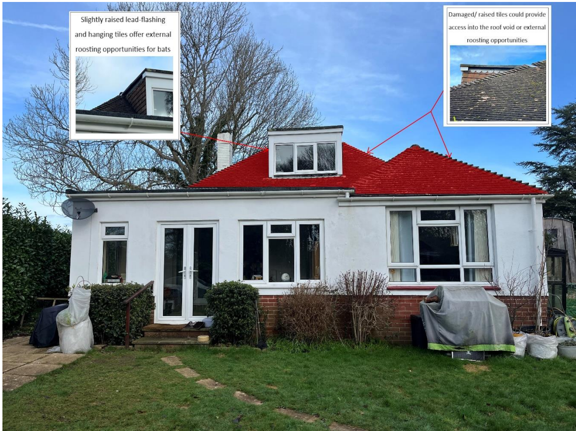
Image 4.3.1.1. Location of potential bat access points and potential external roost locations on the south elevation of the bungalow.
