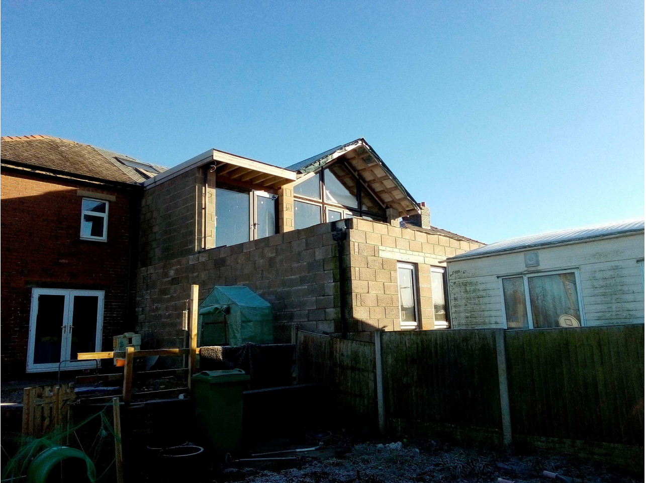
Fig. 2: Looking towards the adjoining house's (number 3) two and single storey rear extensions
