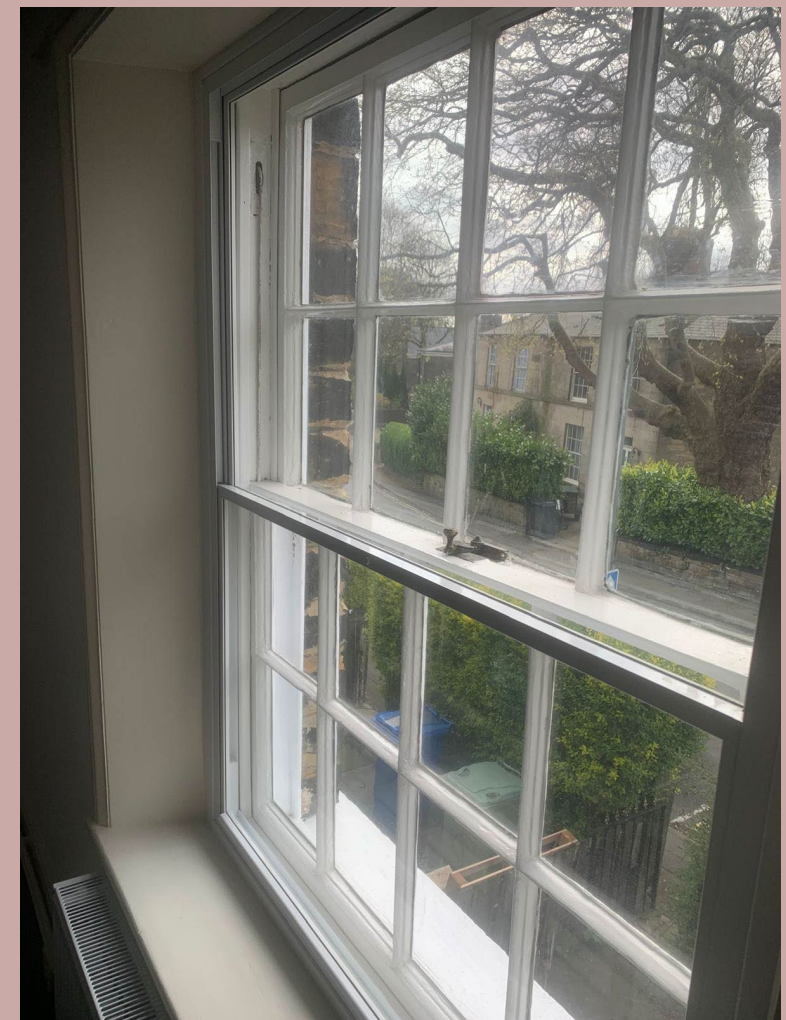
Secondary Glazing in First Floor Sash Window
