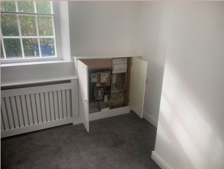
Living room fuse housing
