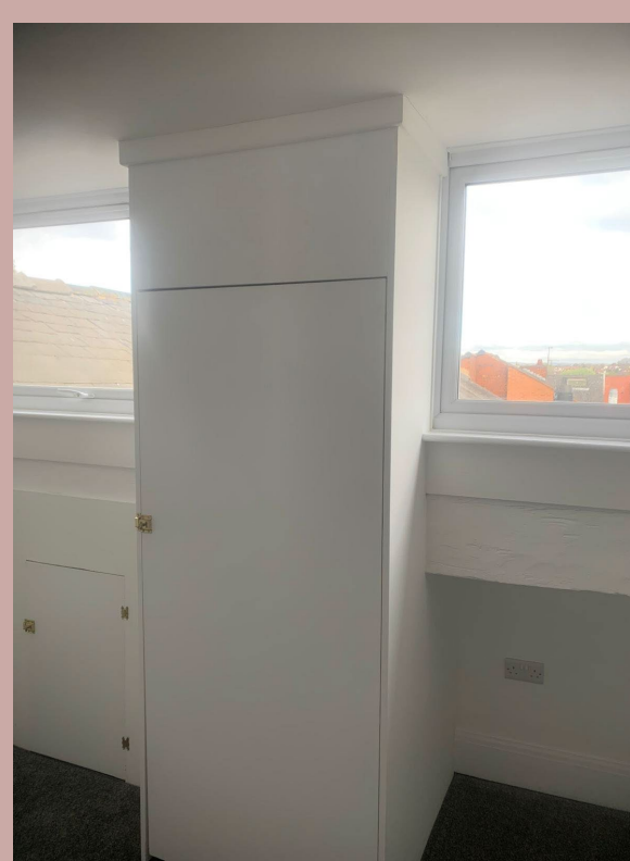
Second floor boiler cupboard
