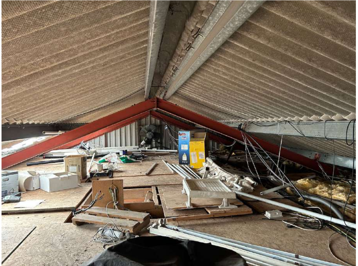
Photograph 6. Void in Building 1
