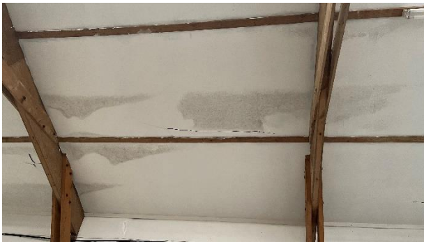
Photograph 12 Cracking to Ceiling of Building B
