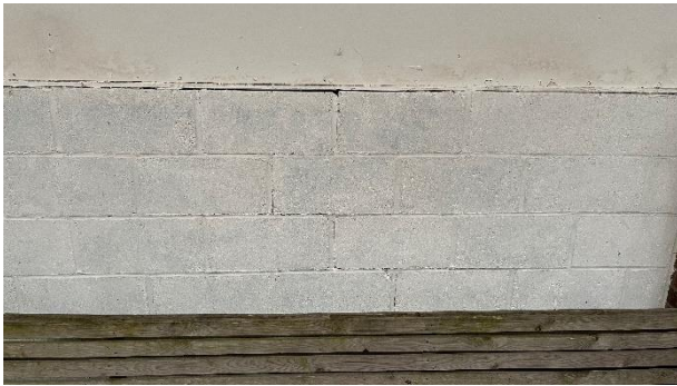
Photograph 10 Cracking to North Elevation of Building B
