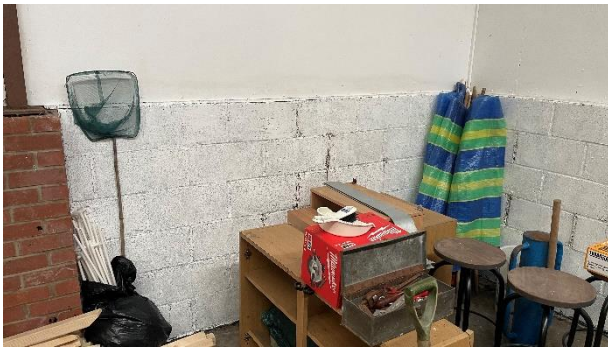
Photograph 11 Paint Cracking to Northeast Corner Building B
