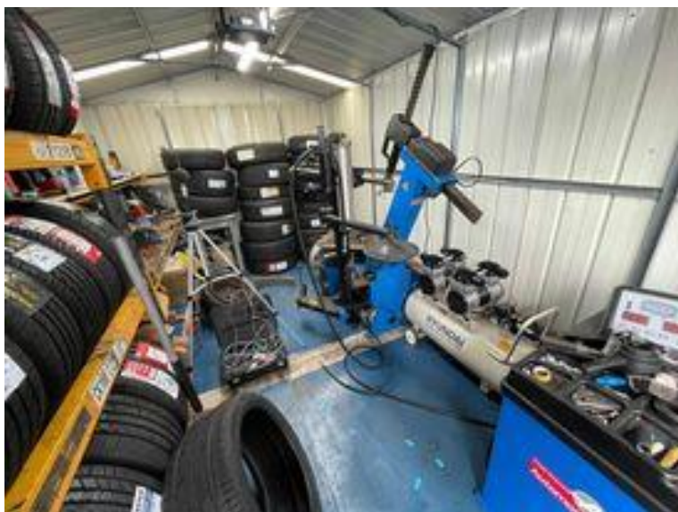
Figure 5.1.1 -Inside the plant room and tire store.
