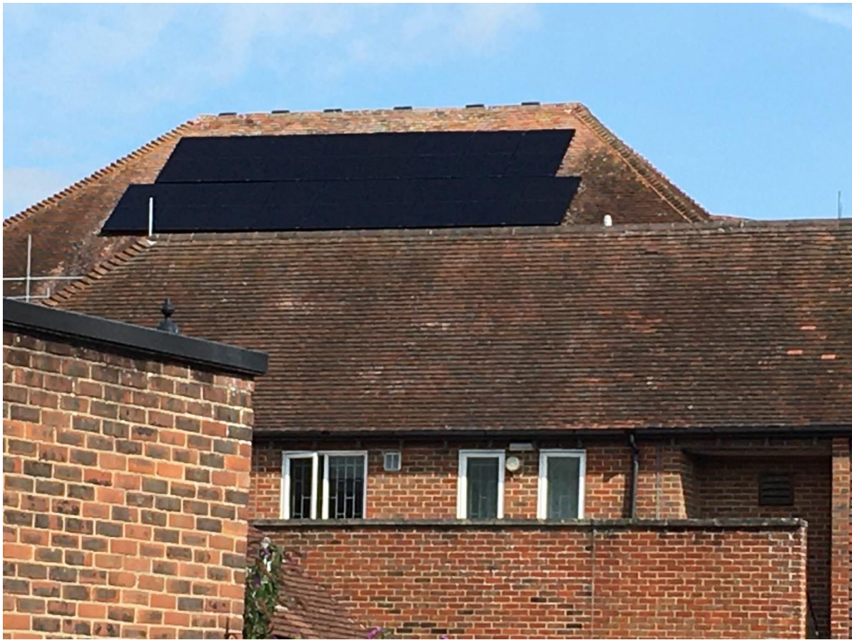
Existing solar panels
