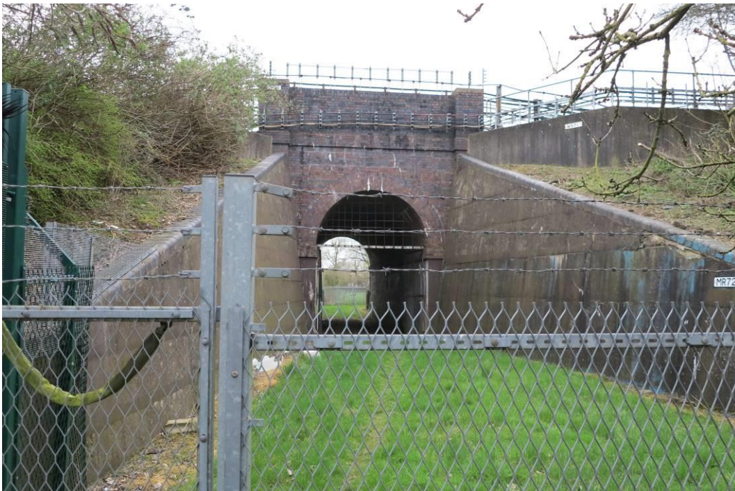
Plate 8. Tunnel through the 1870s' railway banking adjacent to the sports hall, originally intended to provide access between the farmstead and surrounding fields to the east/north-east
