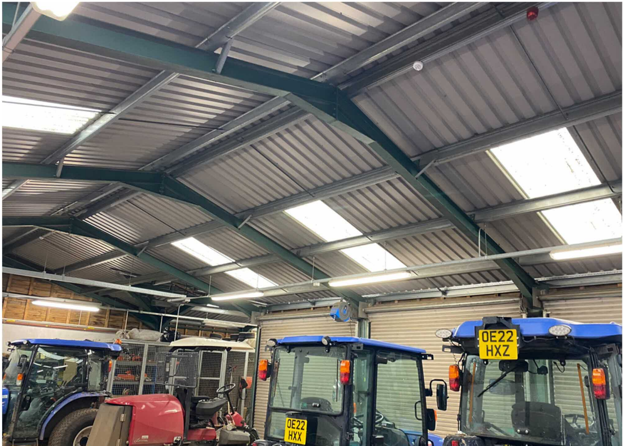
Photograph 5 – internal view showing the arrangement of roof members of the MTS Grounds Maintenance building.
