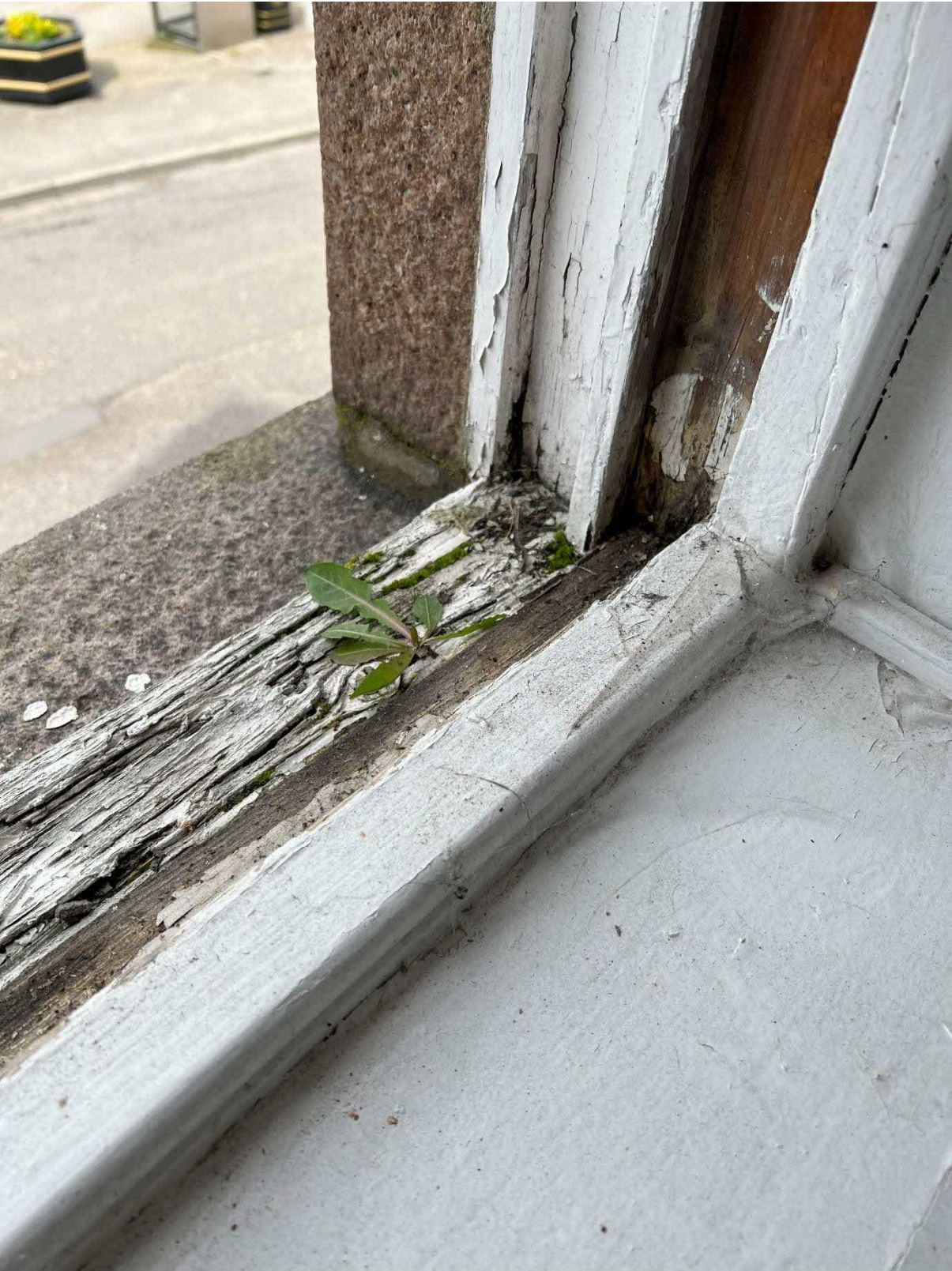
Photo 5 : Example of heavily decayed bottom rail and cill to timber sash and case window to side of building.
