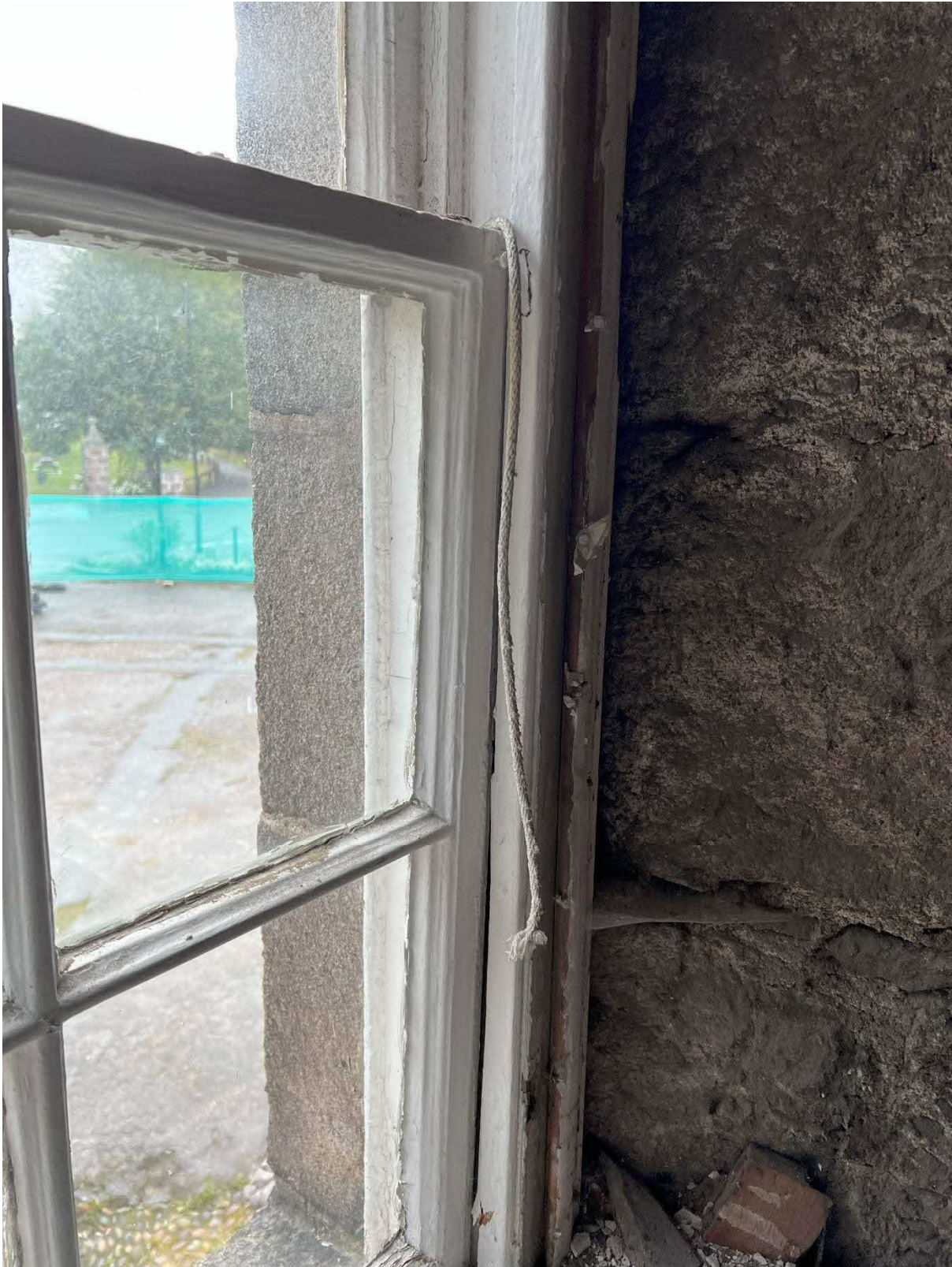
Photo 15 :Example of perished window sash with flaking paint and broken sash cord to timber sash and case window to front of the building.
