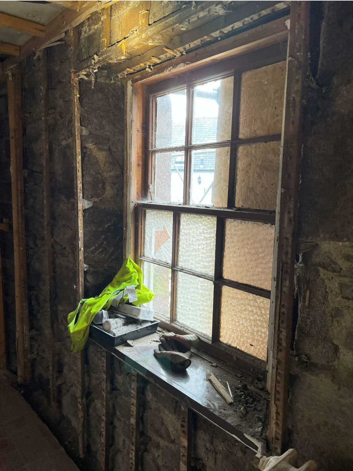
Photo 6 : Example of unfinished and insecure timber sash and case window to rear of building.
