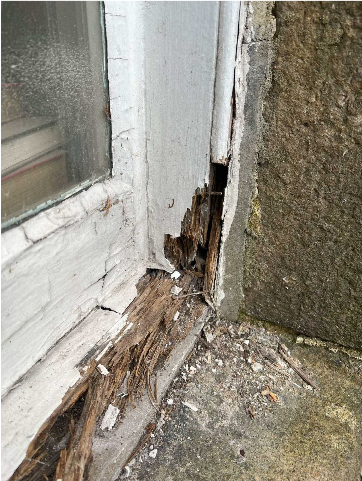
Photo 7 : Example of heavily decayed bottom rail and cill to timber sash and case window to front of building.
