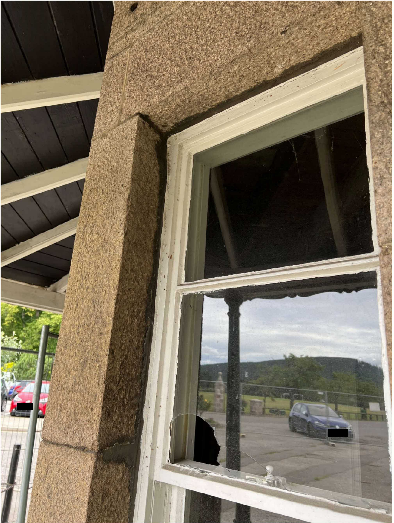
Photo 27 : Example of heavily overpainted window to front of building.
