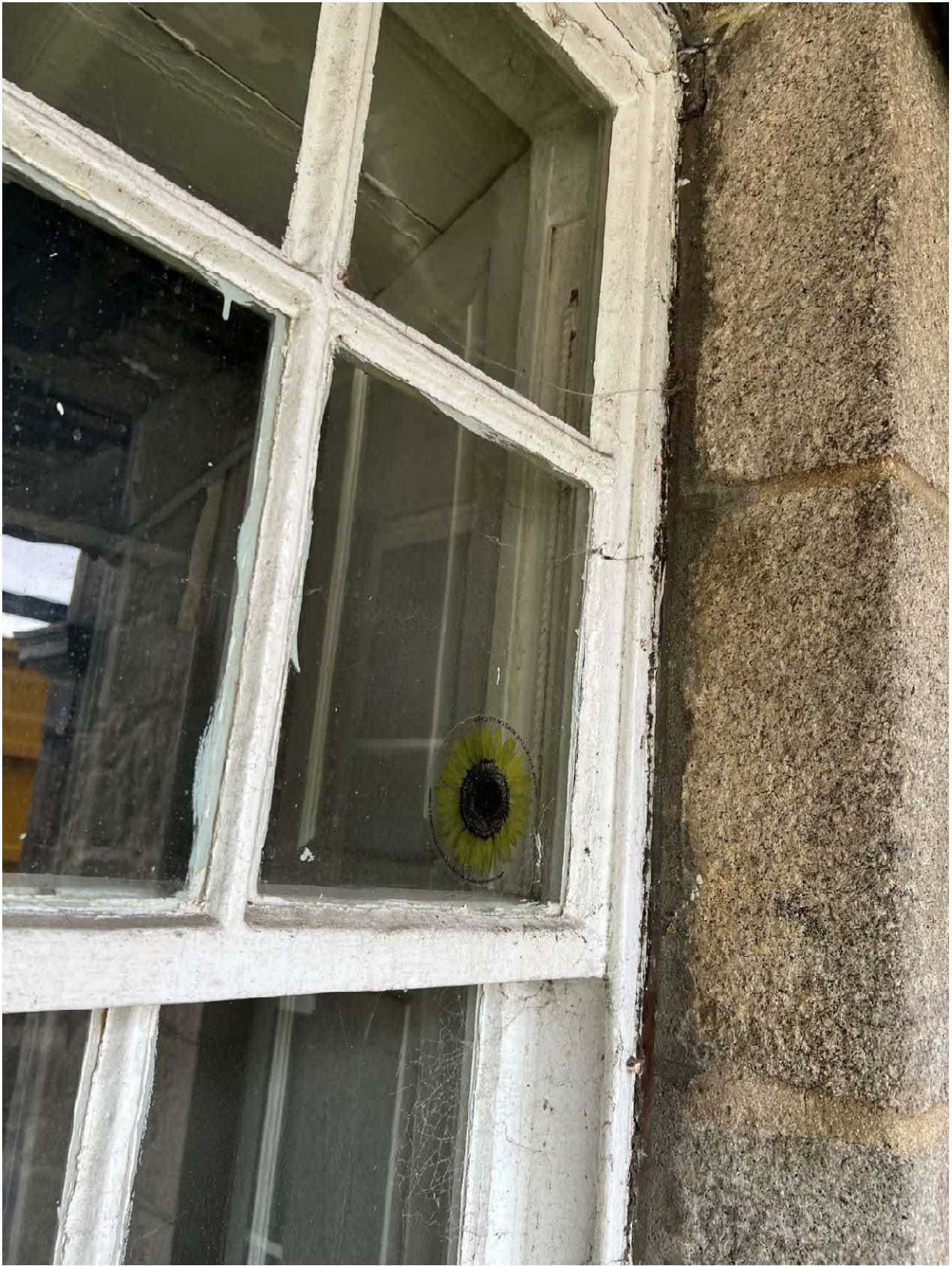
Photo 26 : Example of heavily overpainted window to front of building.
