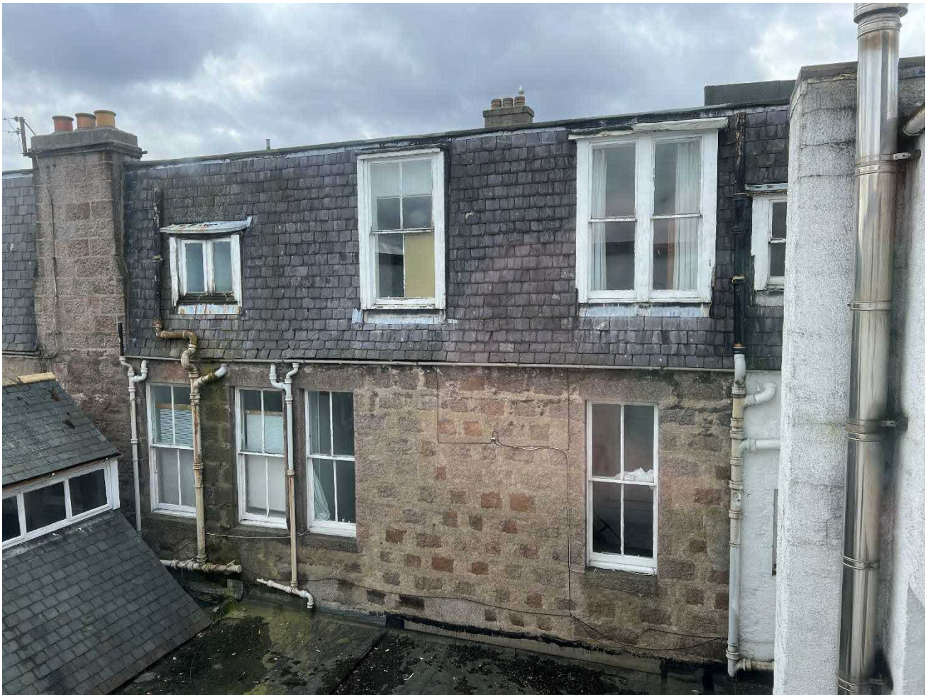
Photo 21 : Photograph of internal rear elevation over courtyard showing the array of window designs and all in extremely poor condition. A mixture of white timber sash and case, white timber casement and white pvc.
