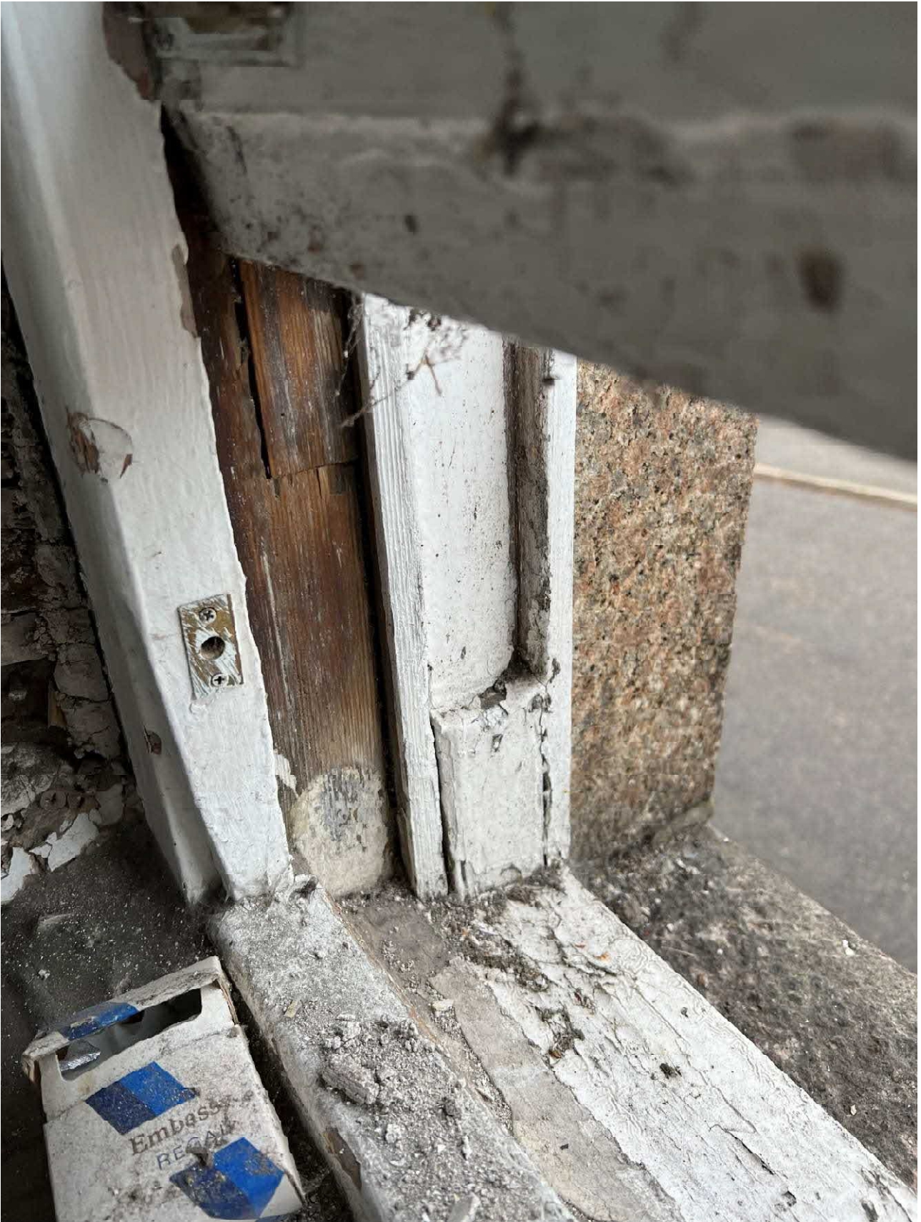
Photo 30 : Example of perished window sash with flaking paint and damaged ironmongery to window on front of the building.
