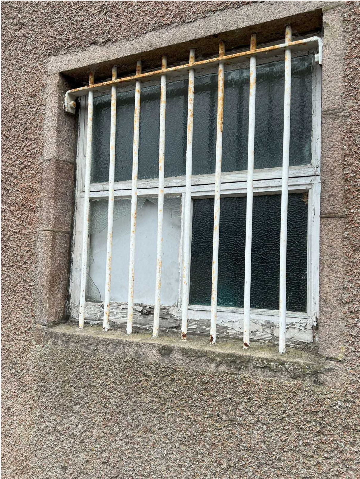
Photo 2 : Example of heavily decayed timber non-sash & case window with security bars
