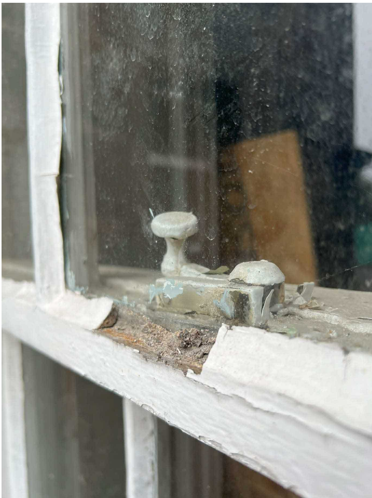
Photo 8 : Example of perished putty sealant with flaking paint and broken ironmongery to timber sash and case window to front of building.
