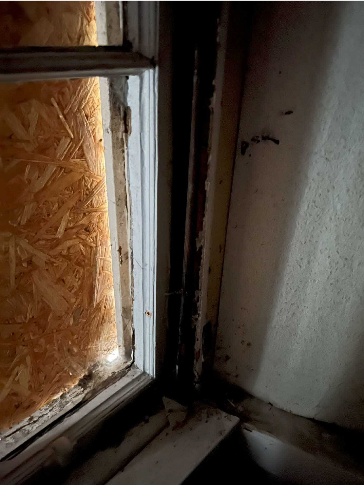
Photo 17 : Example of heavily decayed timber sash and case windows to front of the building damaged by water ingress.
