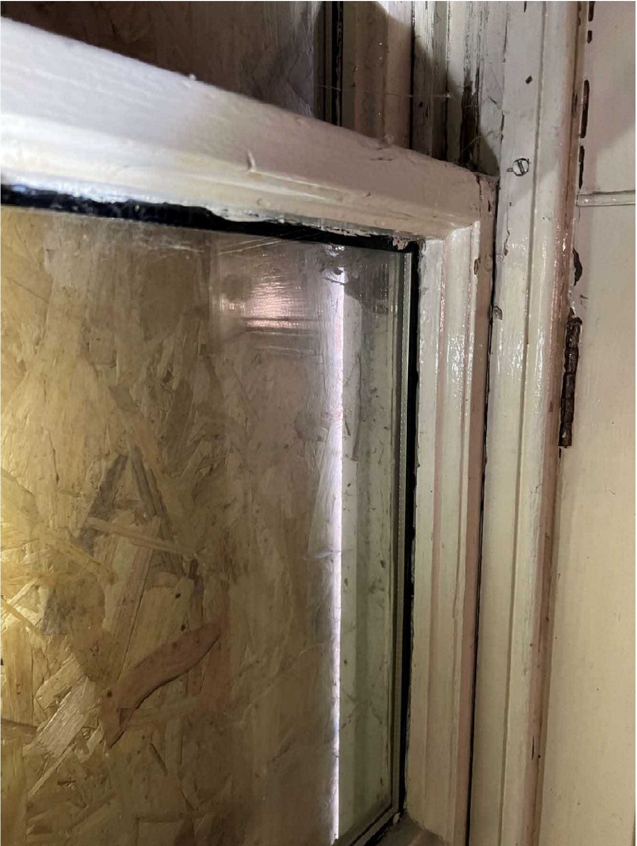
Photo 24 : Photograph of an original sash and case window which has had the glazing replaced with double glazed units and is rotten and heavily overpainted.
