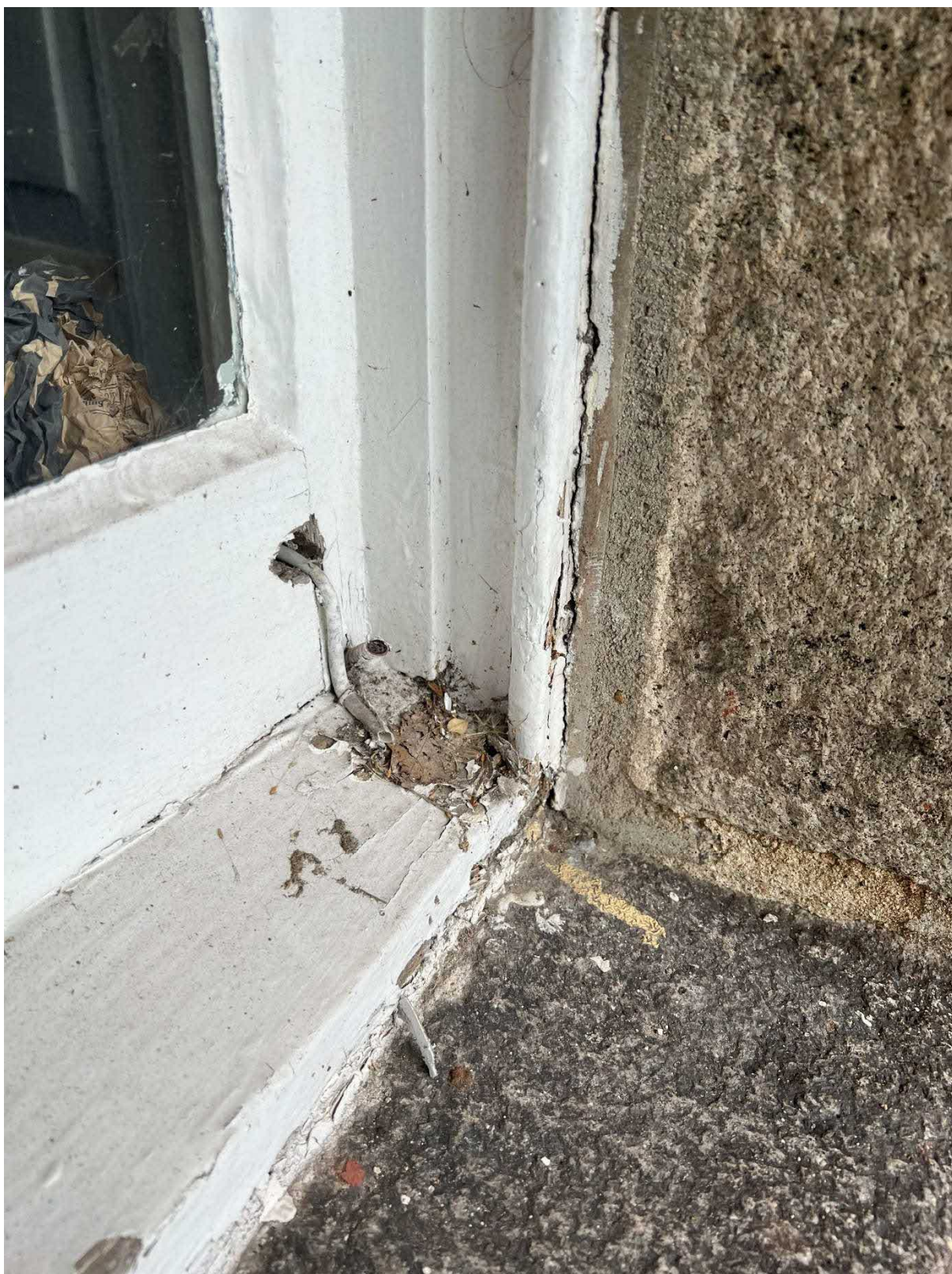
Photo 9 : Example of damaged window bottom sash and decayed bottom rail and cill to timber sash and case window to front of building.
