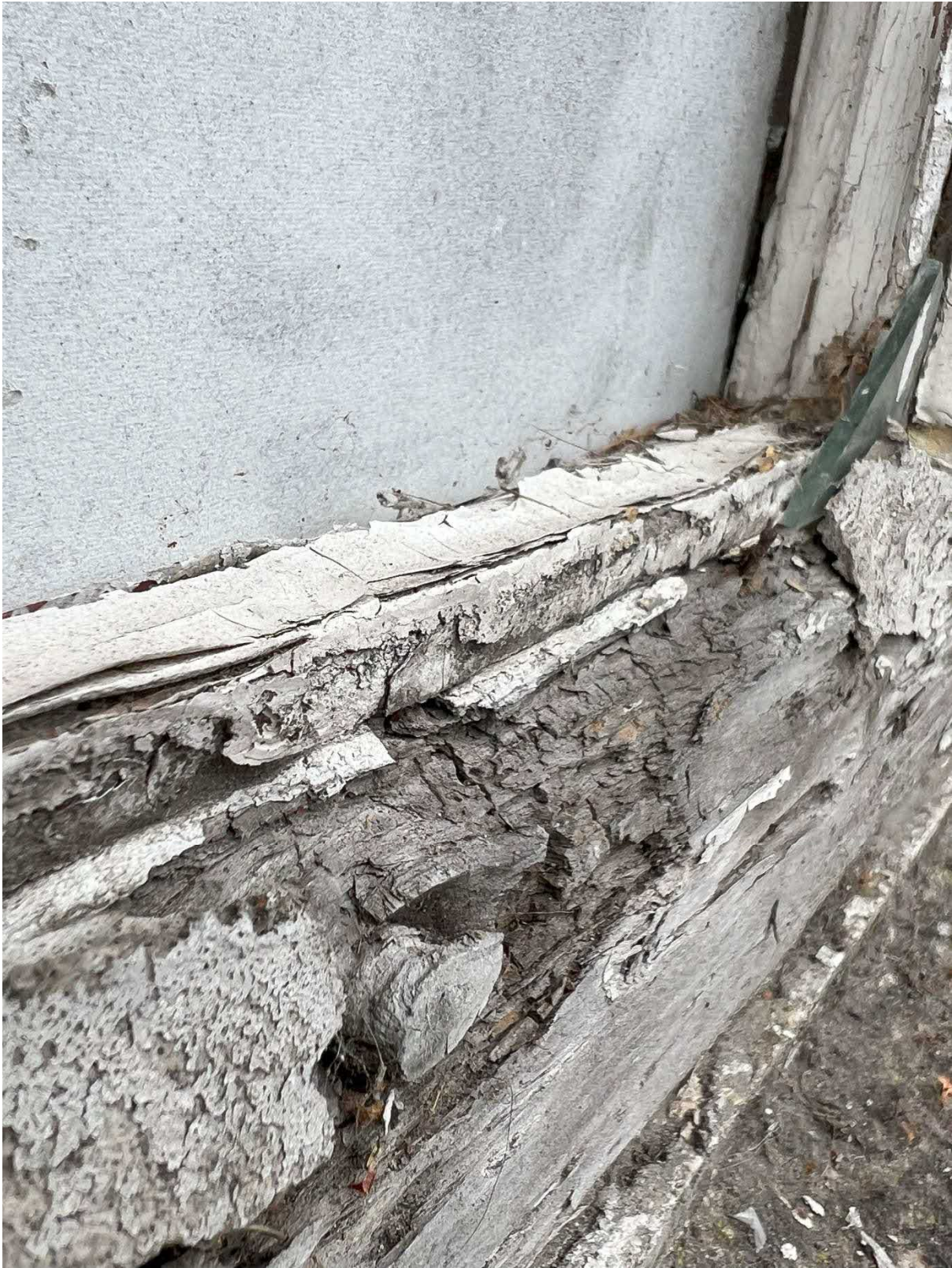
Photo 3 : Example of heavily decayed window frame / cill typical of various windows
