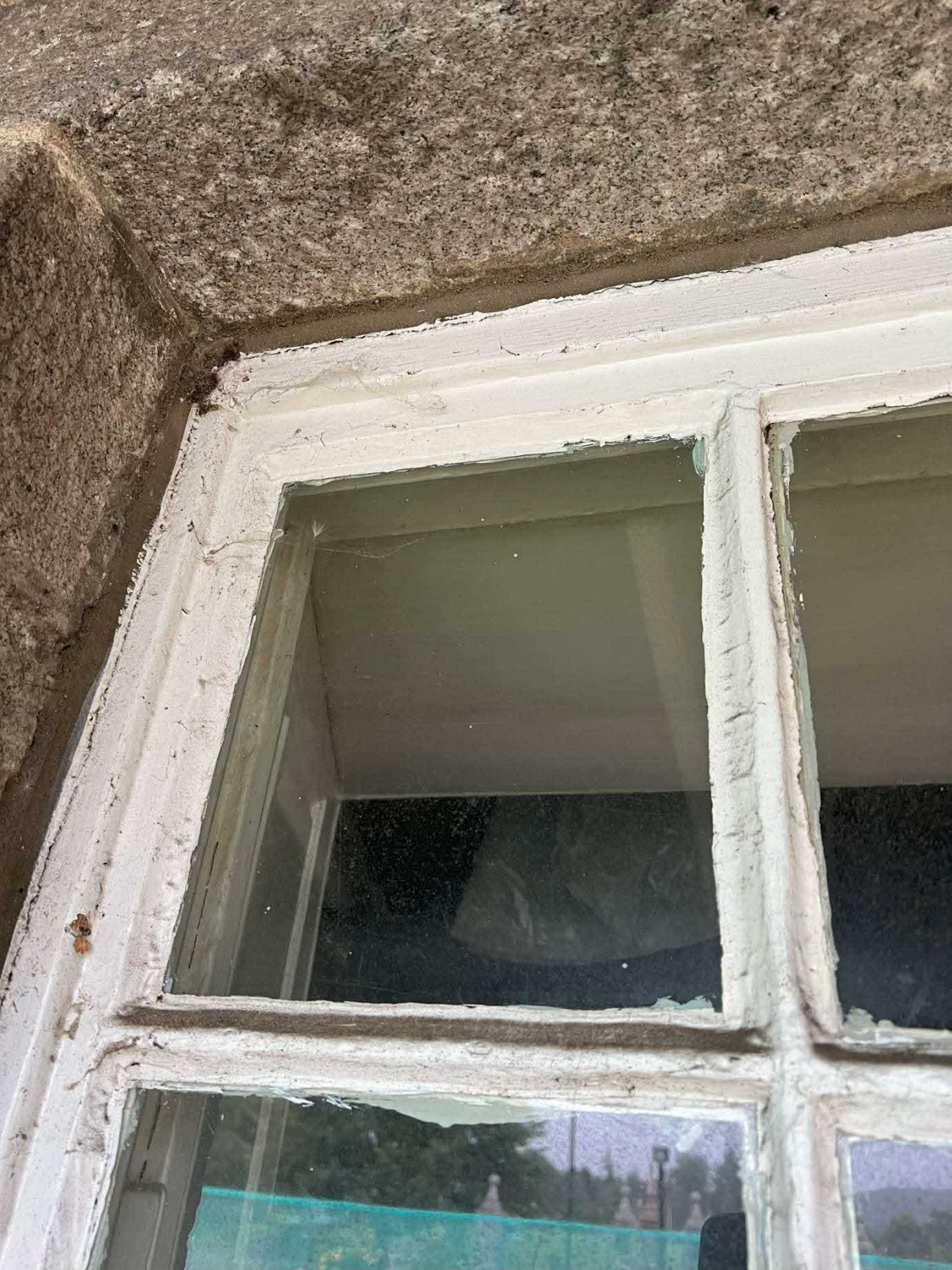
Photo 1 :Example of overpainting to window including astragals and putty sealant
