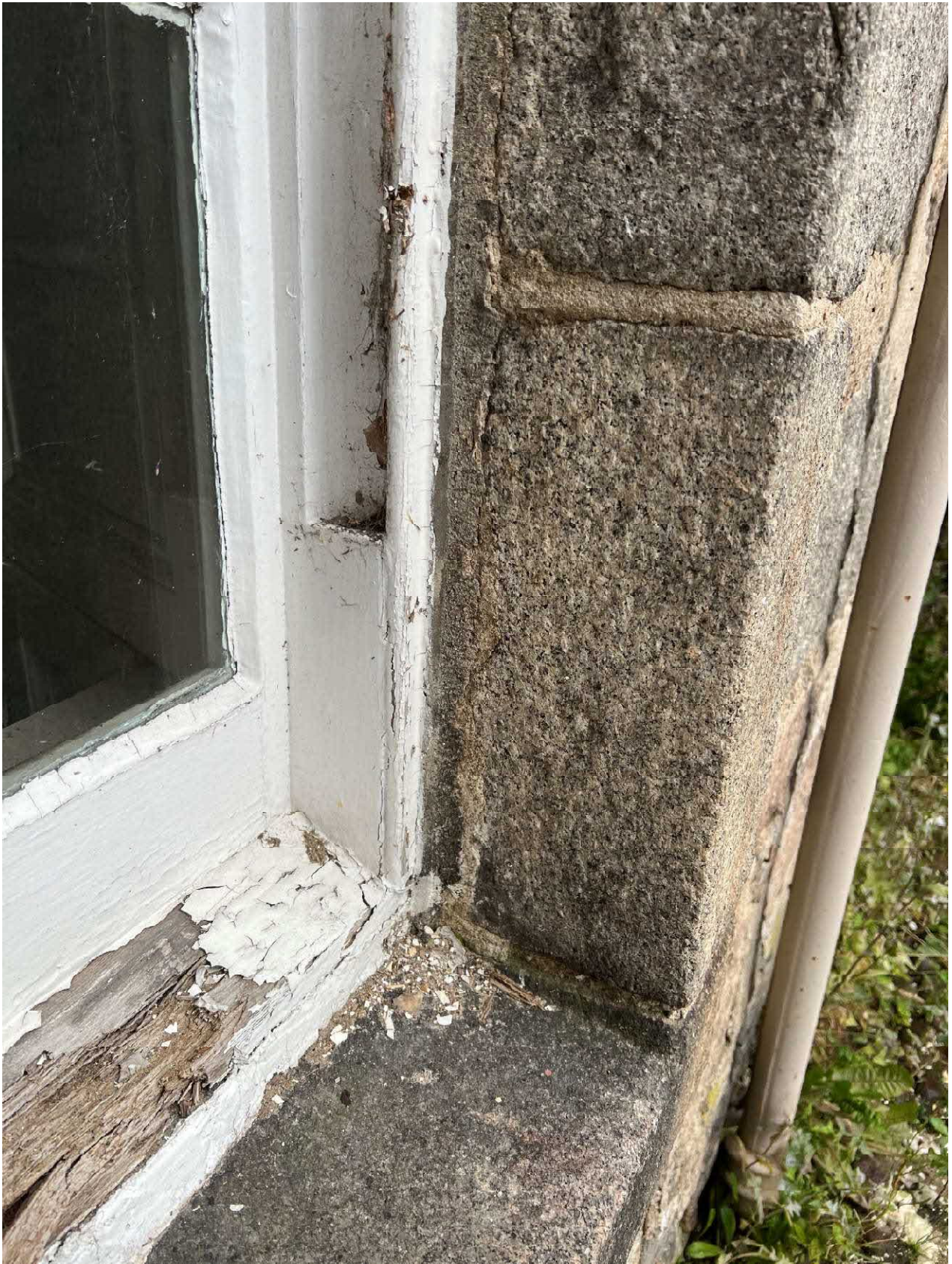
Photo 28 : Example of heavily decayed cill and paint bubbling and flaking along with overpainting and failed putty sealant to window on front of building.
