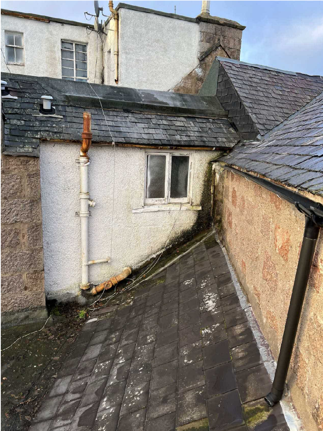
Photo 20 : Example of rotten timber window to rear bedrooms at rear of building.
