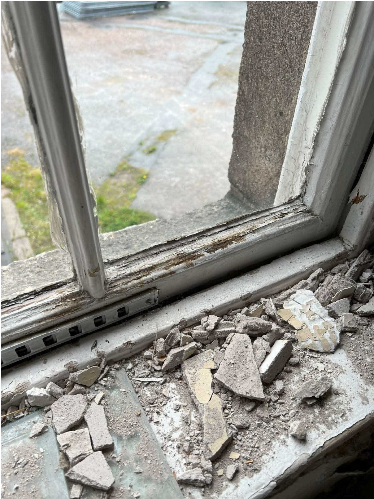
Photo 16 : Example of perished window sash with flaking paint and ironmongery and non-original permanent ventilator that has been fitted to timber sash and case windows to front of the building in attempt to prevent condensation.
