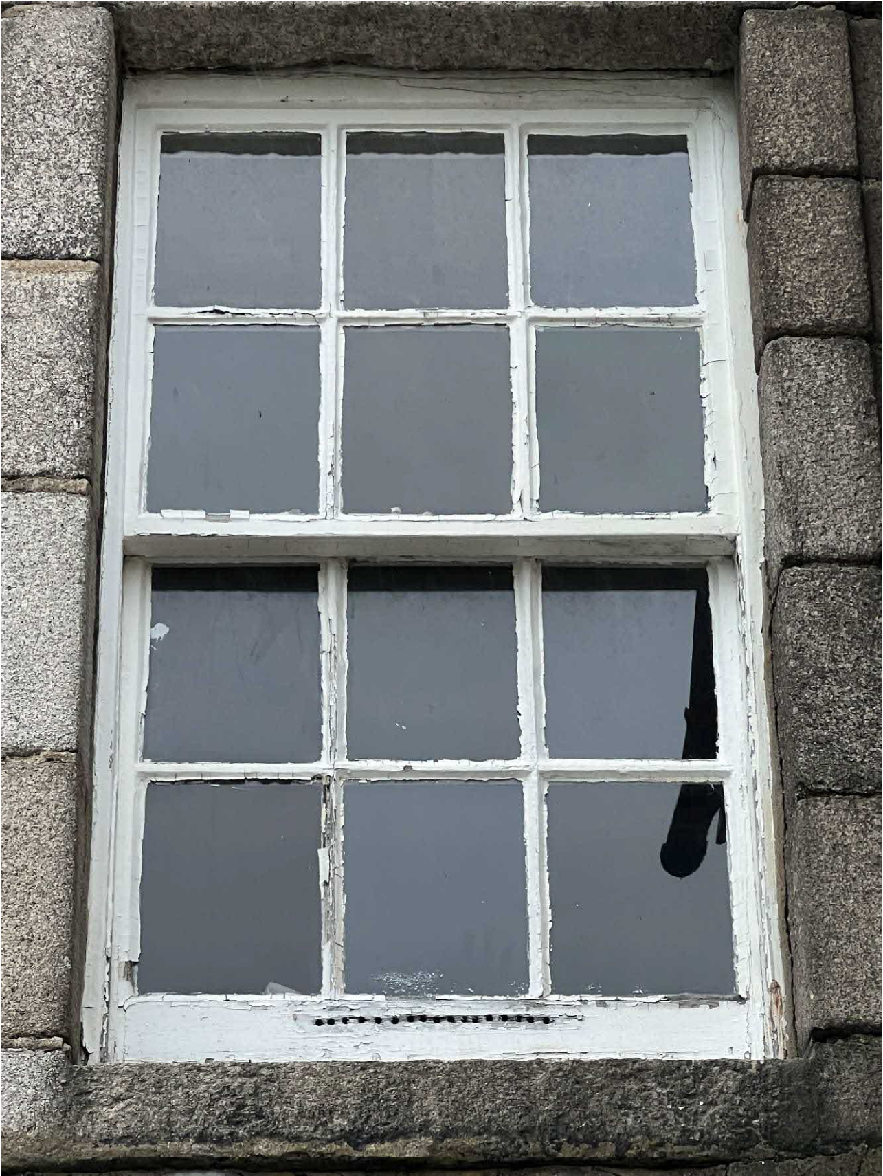
Photo 29 : Example of overpainted window with flaking paint and non-original permanent ventilator that has been fitted in attempt to prevent condensation at front of building.
