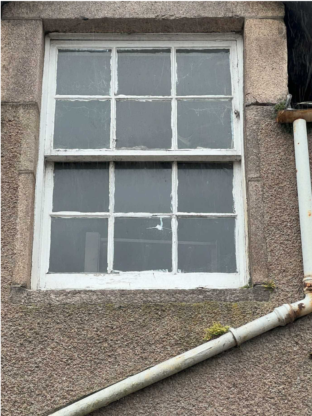
Photo 18 : Example of overpainting to window including astragals and putty sealant to timber sash and case window to side of building.
