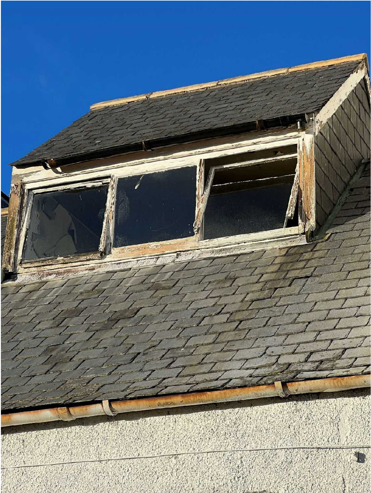
Photo 19 : Example of rotten rear dormer windows over kitchen area to rear of building.
