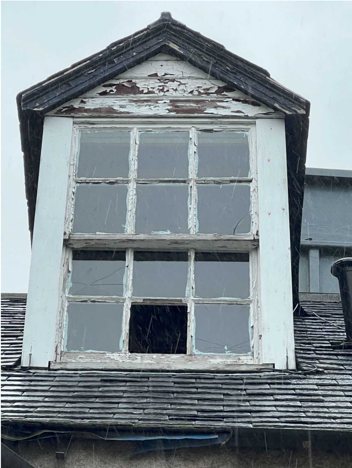
Photo 12 : Example of heavily decayed timber sash and case dormer window to front of building.
