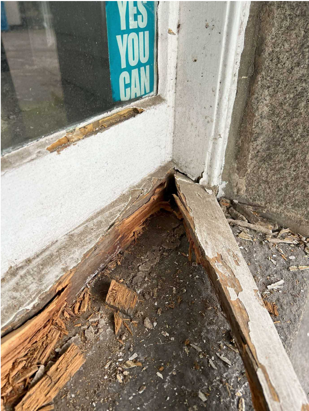
Photo 11 : Example of perished putty sealant and broken window bottom and cill to timber sash and case window to front of building.
