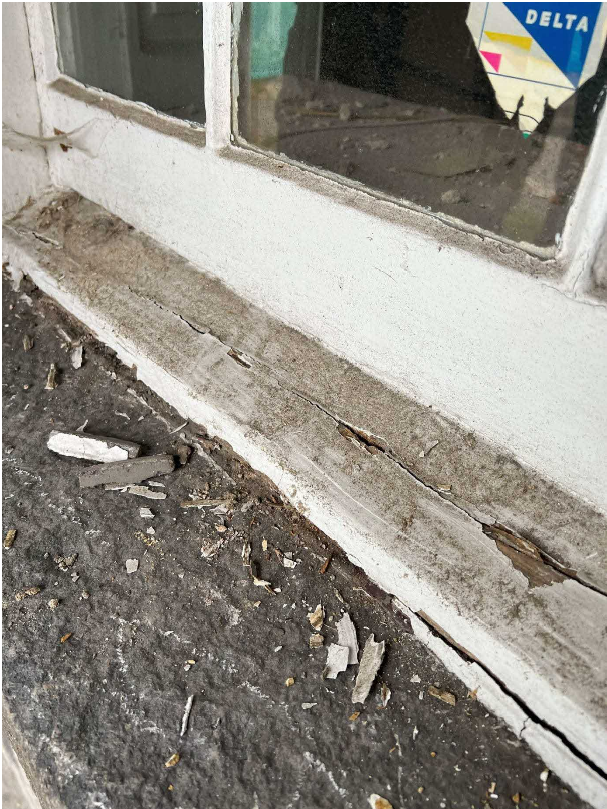
Photo 10 : Example of damaged window bottom sash and decayed bottom rail and cill to timber sash and case window to front of building.
