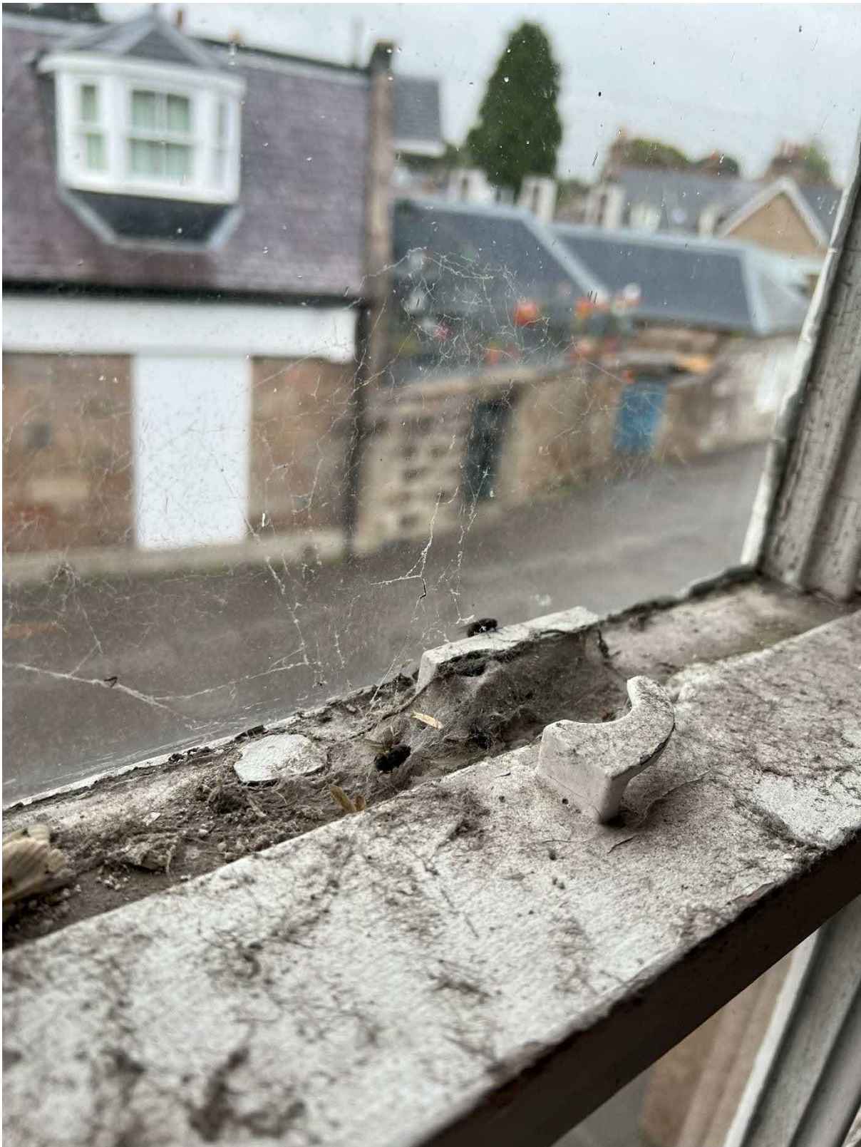
Photo 13 : Example of perished putty sealant with flaking paint and broken ironmongery to timber sash and case window to side of building.
