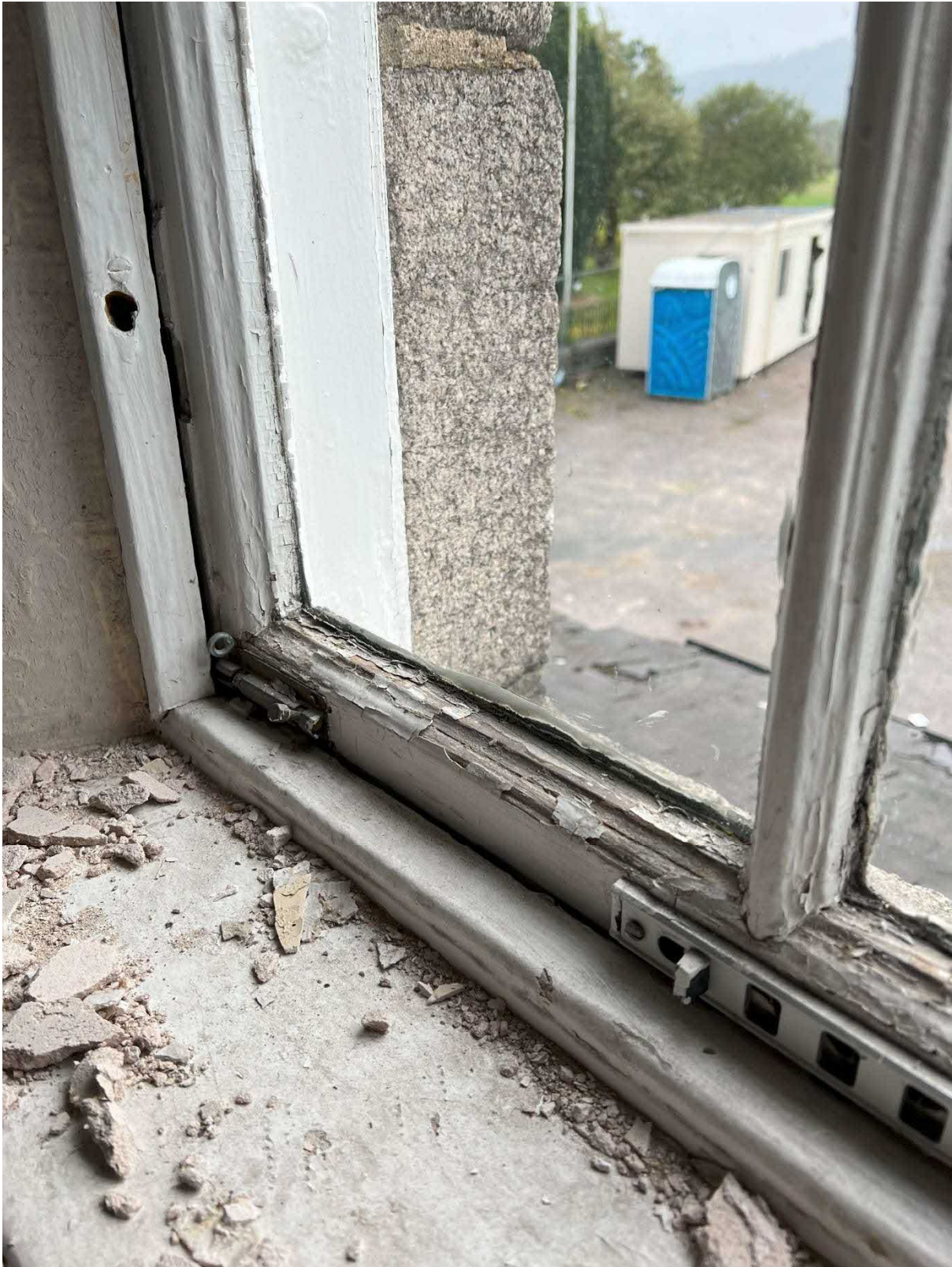
Photo 14 : Example of perished window sash with flaking paint and ironmongery and non-original permanent ventilator that has been fitted to timber sash and case windows to front of the building in attempt to prevent condensation.
